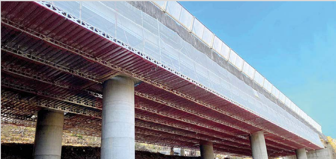
A temporary structure 22 m wide and 250 m long made of 25 cm aluminum beams set up with the FLYRAIL system
